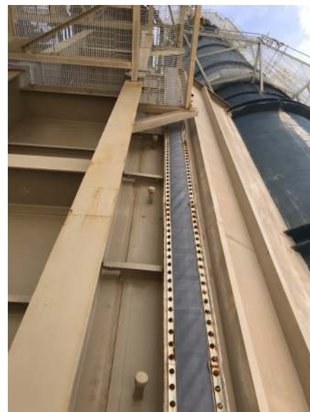
Figure 1: Heat Recovery Unit at Stack
