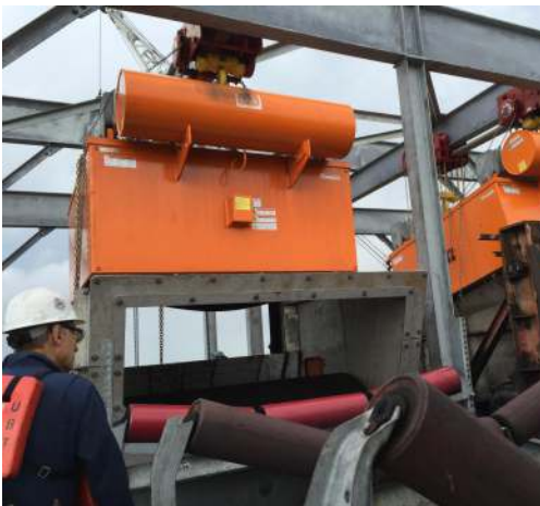
Figure 1: Magnetic separators used to remove scrap metal from the material at the transfer.
