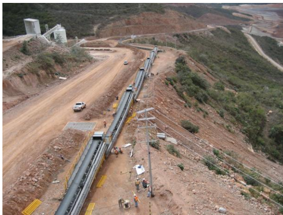
Looking down the Overland Path: From the tail of TB 27, the agglomerating conveyor
