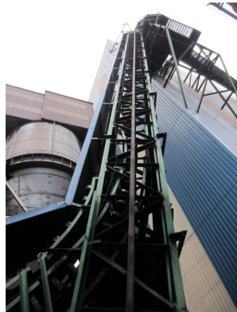
The DSI Sandwich conveyor replaced a problematic pocket belt system eliminating carry back and clean up problems by scraping belts clean.
